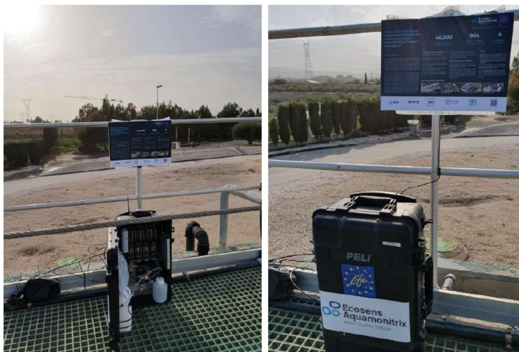
Figure 4.3.2: Device deployment in Alcantarilla wastewater treatment plant (WWTP) (Source: Martínez et al., 2020)
