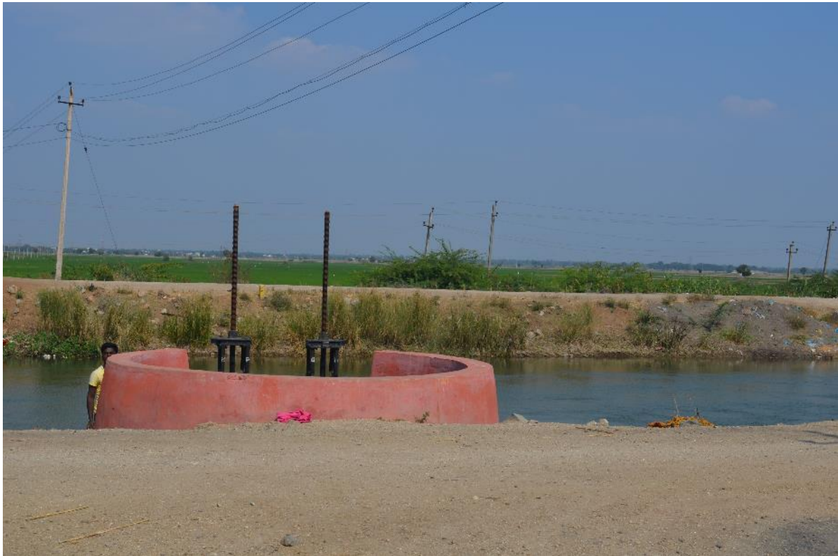
Figure 2-3: Intake well at LLC
