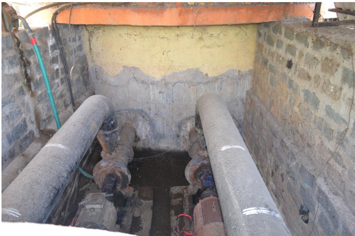
Figure 2-13: Pump infrastructure supplying treated used water from Ananthapur UWTP to Janaki Corporation
